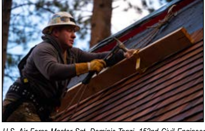
U.S. Air Force Master Sgt. Dominic Tanzi, 152nd Civil Engineer Squadron operations management noncommissioned officer in charge, hammers a nail into a support beam at the Tallac Historical Site, South Lake Tahoe, Calif., October 21, 2021. Tanzi has been training and working on projects with the U.S. Forest Service at the Tallac Site since he joined the unit in 1998. (U.S. Air National Guard photo by Airman 1st Class Thomas Cox)
