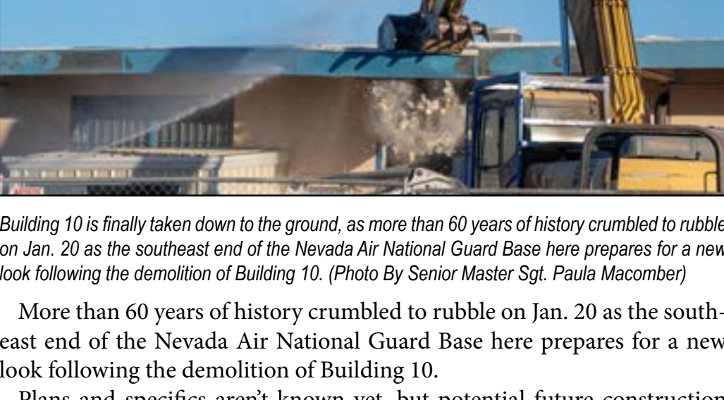
Building 10 is finally taken down to the ground, as more than 60 years of history crumbled to rubble on Jan. 20 as the southeast end of the Nevada Air National Guard Base here prepares for a new look following the demolition of Building 10. (Photo By Senior Master Sgt. Paula Macomber)
