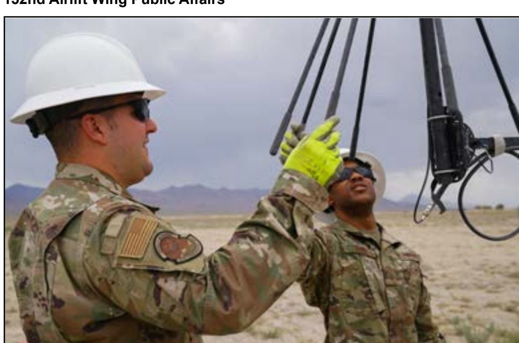
U.S. Air Force Staff Sgt. John Gunn, right, and U.S. Air Force Tech. Sgt. Marvin Drake, both Joint Incident Communications Capability team members with the 152nd Communications Flight, take down an antenna at Fallon Range Training Complex, Nev., June 24, 2021. The Airmen were providing communication support for Exercise Resolute Hunter, a joint exercise with the Nevada Air National Guard, Nevada Army National Guard, and the Navy. (U.S. Air National Guard Photo by Airman 1st Class Michelle Brooks)
