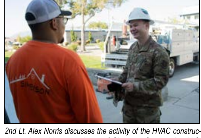
2nd Lt. Alex Norris discusses the activity of the HVAC construction project with an employee of Simerson Construction LLC, prime contractor, during an unscheduled site walk to validate daily development in accordance with the provided progression reports from the contractor.
